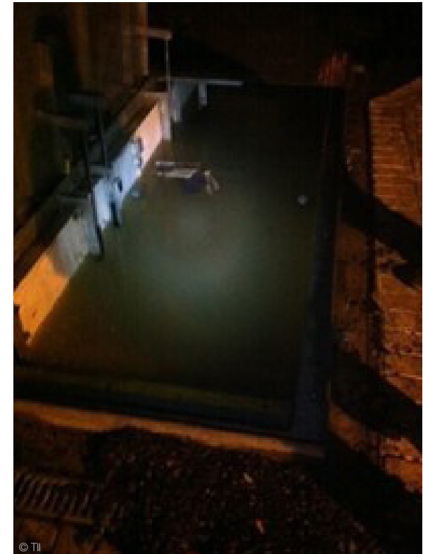
Figure 23 Flooded Luas substation
