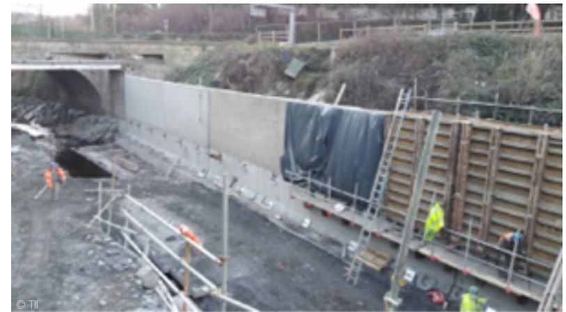
Figure 25 Erosion on N11 along the river Dargle
